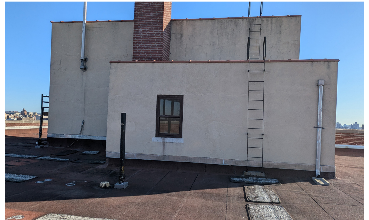
13: View of South Elevation at Bulkhead A and Elevator Machine Room (beyond)
