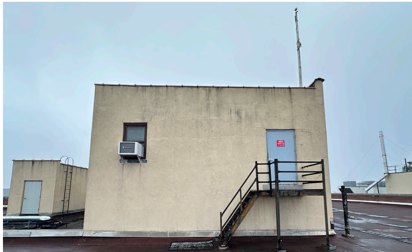
10: View of West Elevation at Elevator Machine Room and Bulkhead B (beyond)
