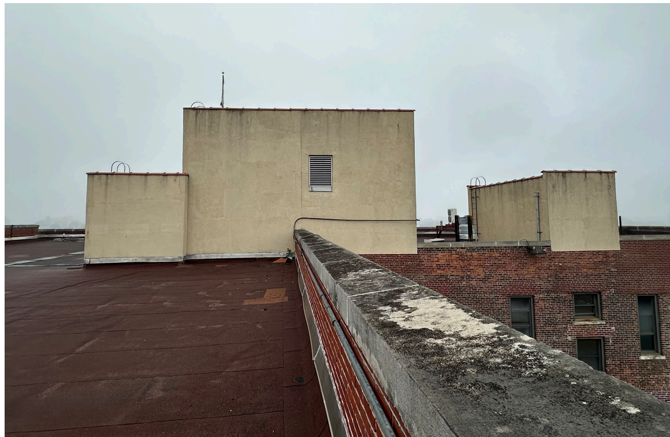
12: View of East Elevation (from left): Bulkhead A, Elevator Machine Room and Bulkhead B
