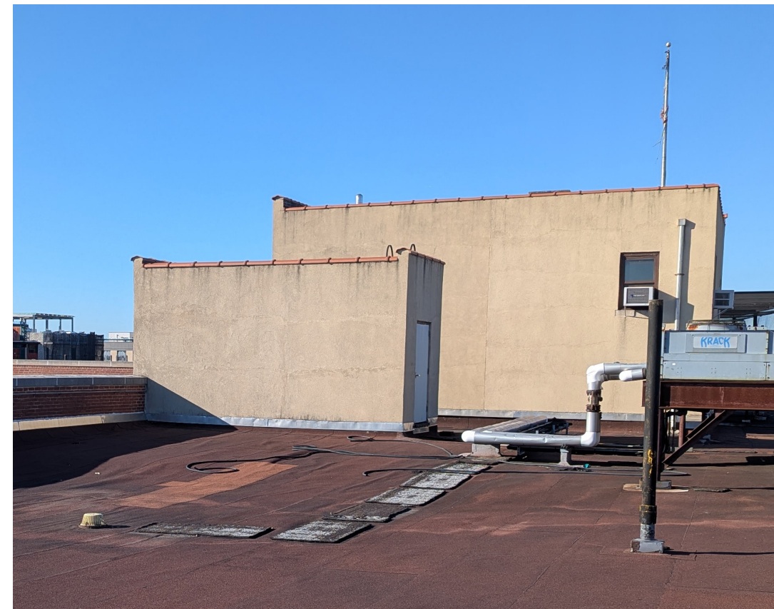
11: View of North Elevation at Bulkhead B and Elevator Machine Room (beyond)
